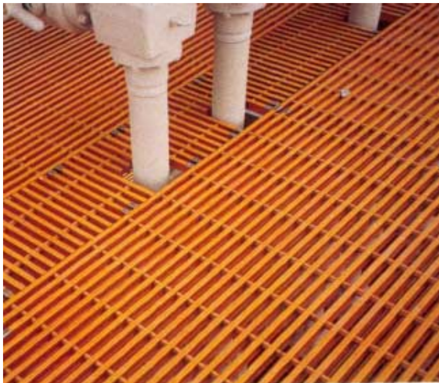
Figure 19. Application of pultruded phenolic gratings on a tension leg platform in the Gulf of Mexico (Courtesy of Strongwell).
