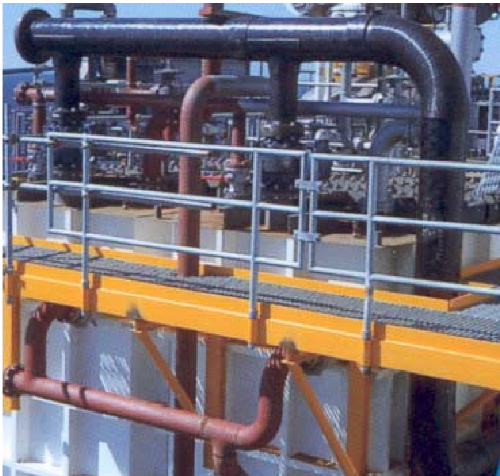
Figure 3. Glass fibre reinforced epoxy pipework on an offshore platform (Courtesy of Ameron BV).
