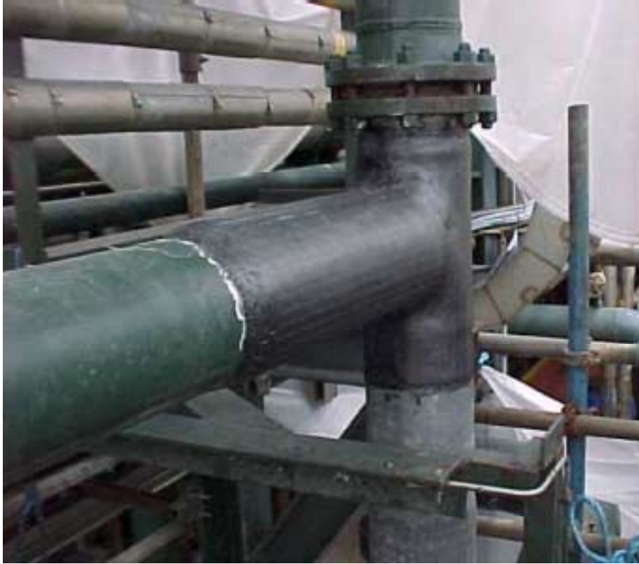
Figure 14. Carbon fibre repair of 14 inch tee joint on a seawater return header (Courtesy of DML).
