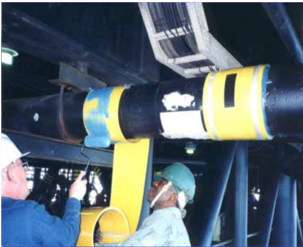
Figure 13. Offshore application of a 'Clockspring' repair to an externally corroded pipe (Courtesy of Clockspring Ltd).
