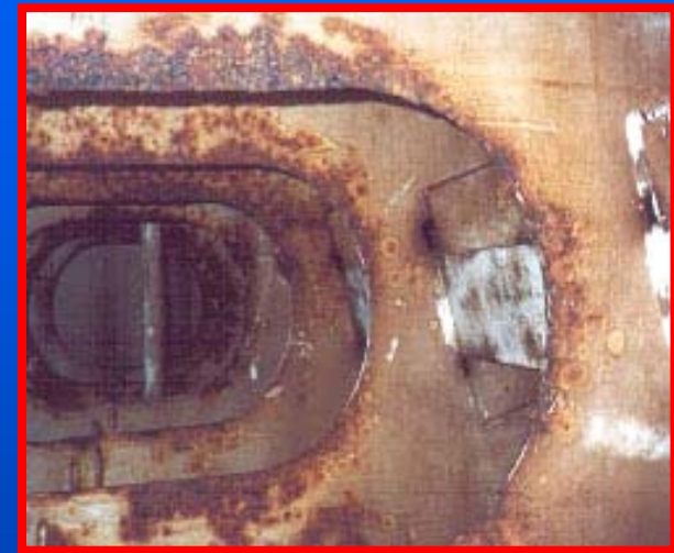
Current Tank Coatings after 36 Months [ERM, Beau Brinckerhoff, 05M]
