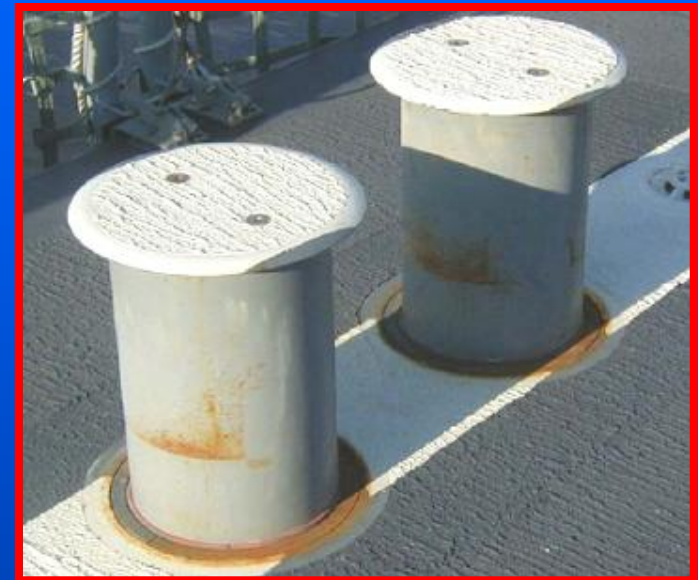
Typical Retractable Bitt Showing Corrosion from Mooring Line Wear and Standing Water
