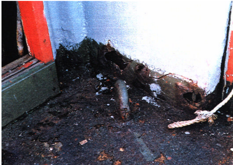
Photograph 1 Corroded accommodation house structure
