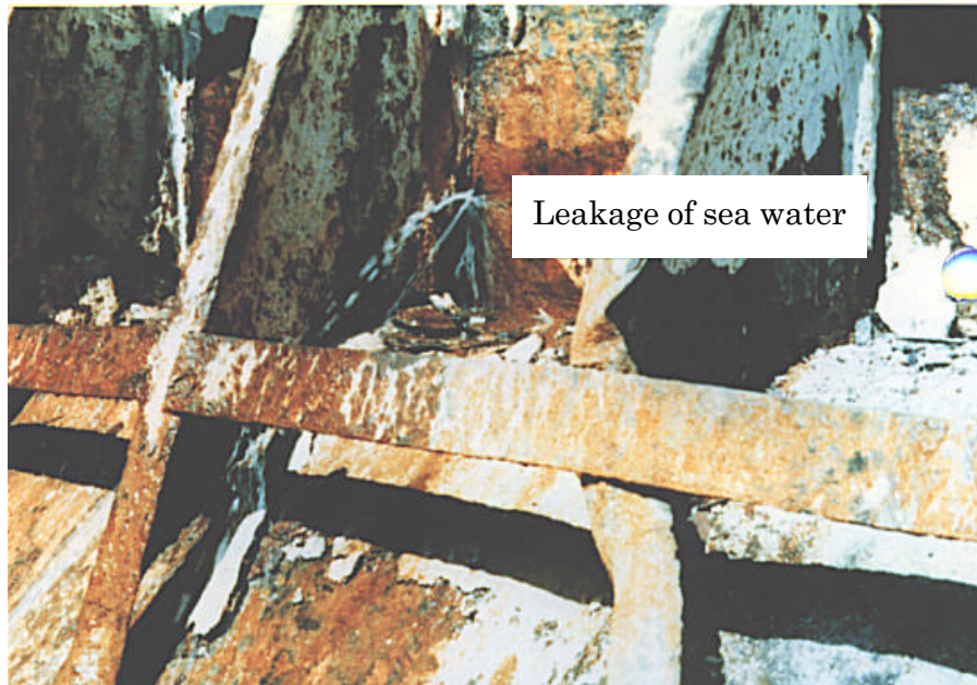
Photograph Leakage from side shell plating due to heavy corrosion
