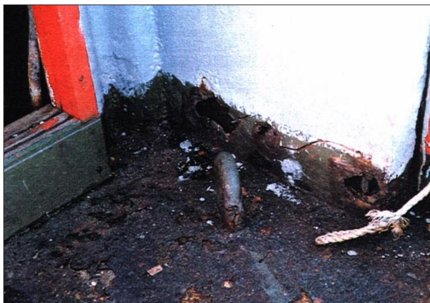
Photograph 1 Corroded accommodation house side structure
