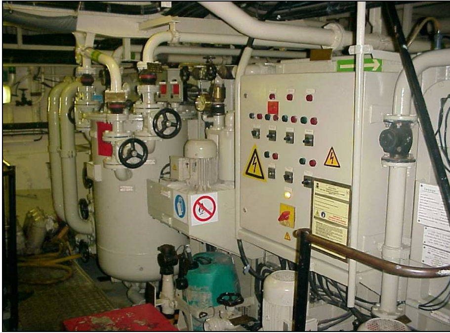
Fig. 6.3 – Photograph of a biological sewage treatment plant.
