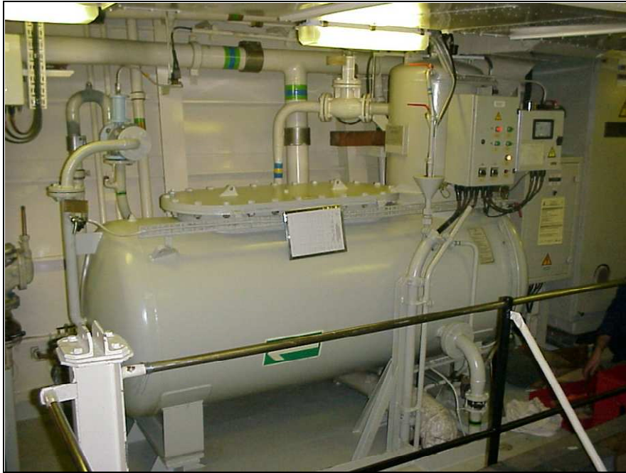
Fig. 6.6 – Photograph of an oily water separator.
