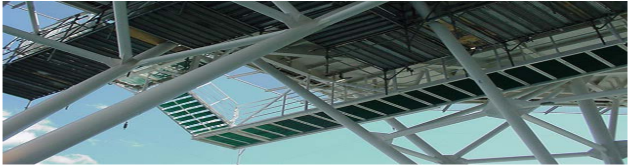
part of the superstructure on an FPSO
