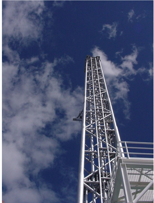
Terra Nova Flare tower
