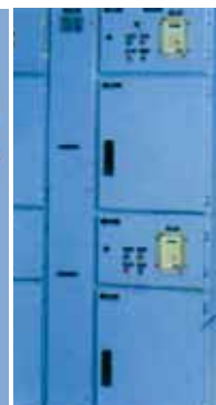
Medium Voltage Cubicles.
