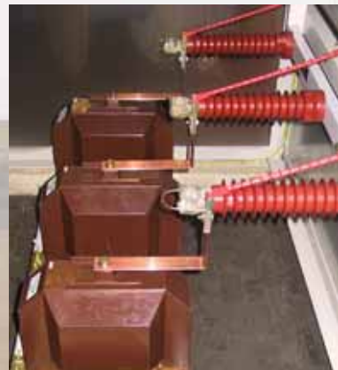
UCL - 24 Voltage transformers for medium voltage cubicles.
