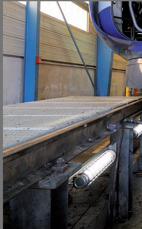
SNCF, VILLENEUVE-SAINT-GEORGES/FRANCE - FOSSES DE VISITE SNCF, VILLENEUVE-SAINT-GEORGES/FRANCE - INSPECTION PITS
